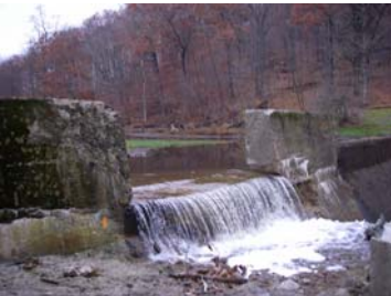
Notched YMCA Camp Dam in Mount Olive
