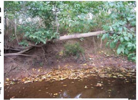
Eroded bank of Walnut Brook.
